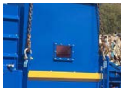
HOPPER VIEW WINDOW
